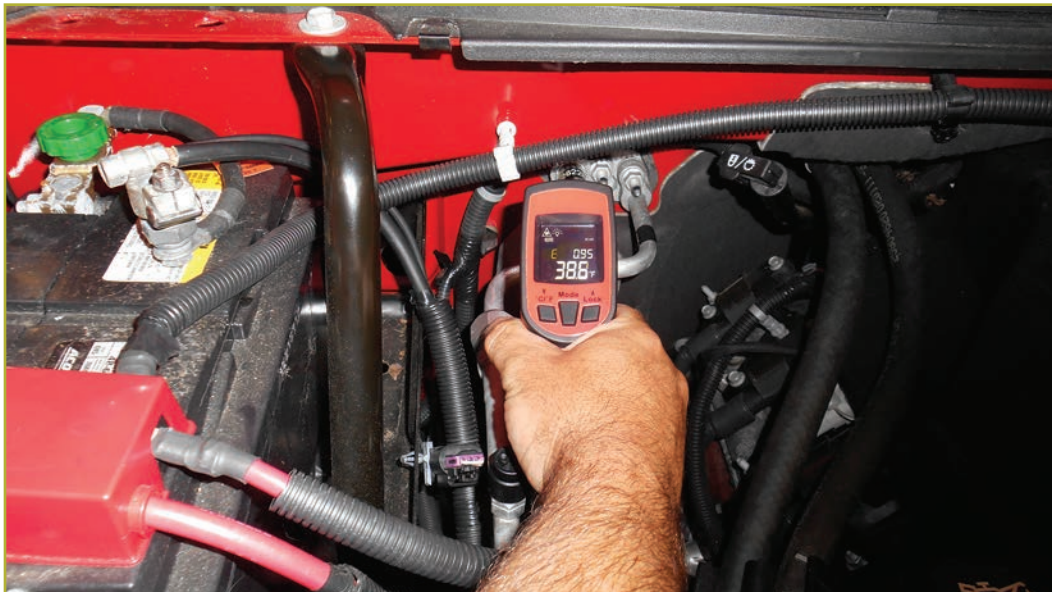
FIGURE 3 —Measure the temperatures of the evaporator inlet and outlet lines as closely as possible to the evaporator. (Courtesy of Dr. John Kershaw)
